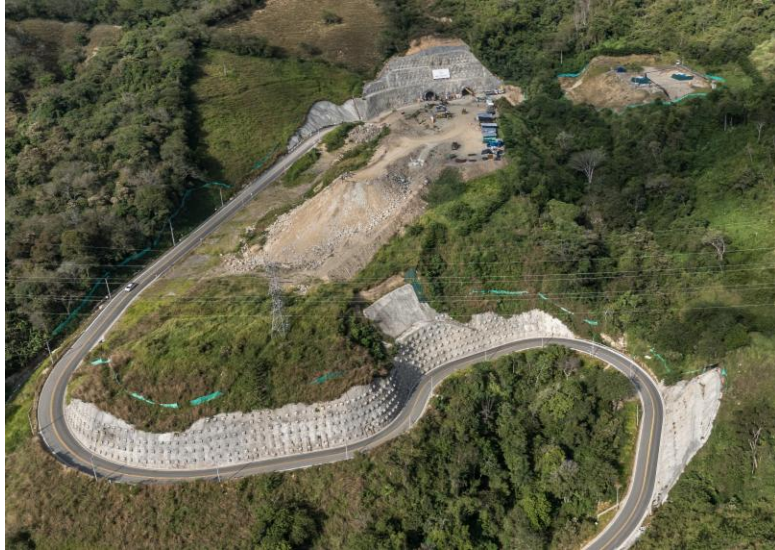
Access roads to the Lower Marmato process facility and accommodation camp now 100% complete
