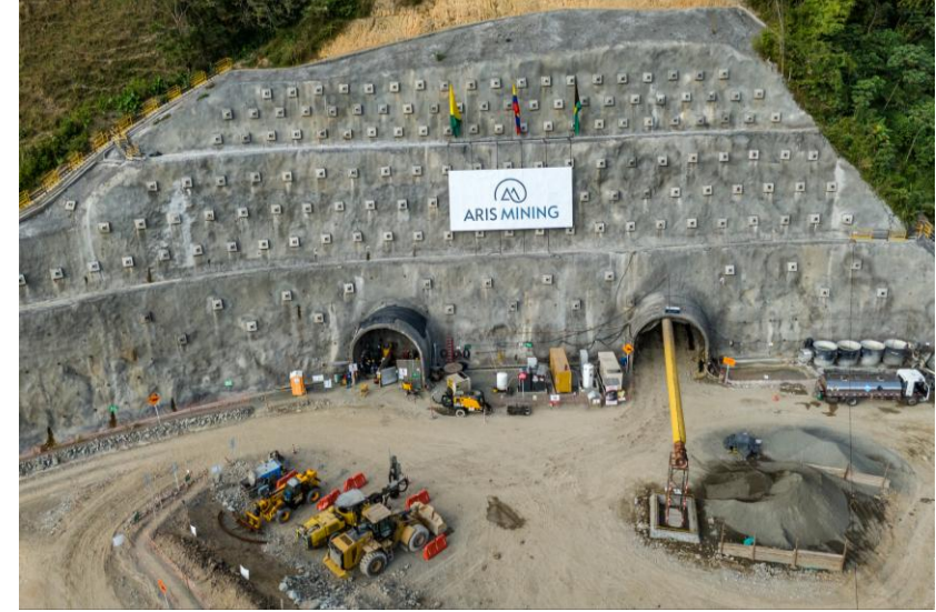
Process plant foundation earthworks 12% ahead of schedule as of the end of February 2025
